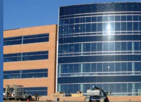
National Energy Center of Excellence
